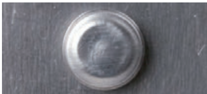
Joint from below – die side
